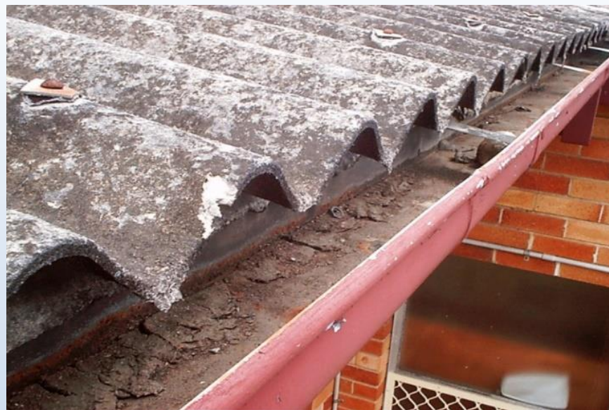
Deteriorating Asbestos Cement Roof Cladding
